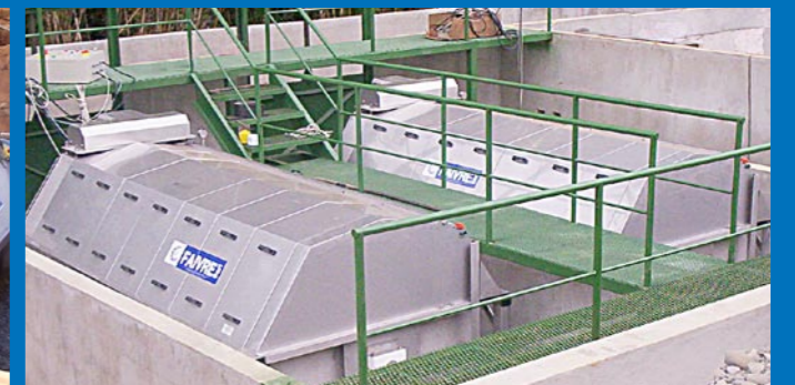
View on 2 filters 28-160 with frame in outlet fish farm
