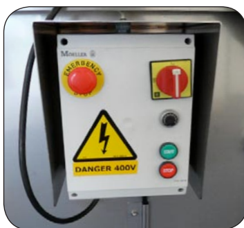
Electrical box with electronic adjustable speed
