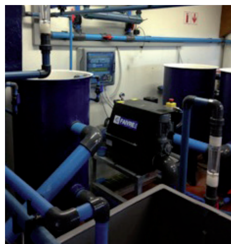
Drum filter model 1-40 with tank ( in sturgeon recirculation system )
