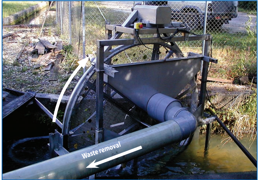
Ø2200 SCREENS: View from the water inlet side (above) View from the water outlet side (above)
